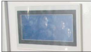
PLC control touch screen panel
